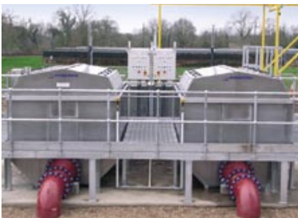
Installation at waste water treatment plant.
